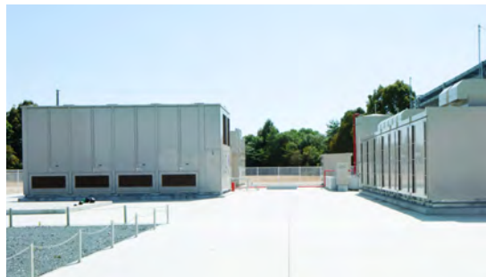
Large-capacity power storage system (Yamaguchi Plant)
