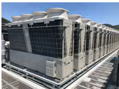
Module-type heat pump chiller (Minase Research Institute)
