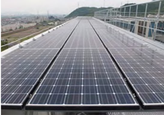
Solar panels (Minase Research Institute)
